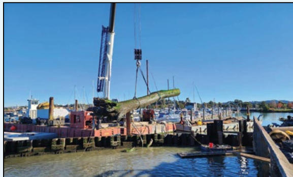
The contractor removed the large tree from below the fishing pier as part of the in-water work.
